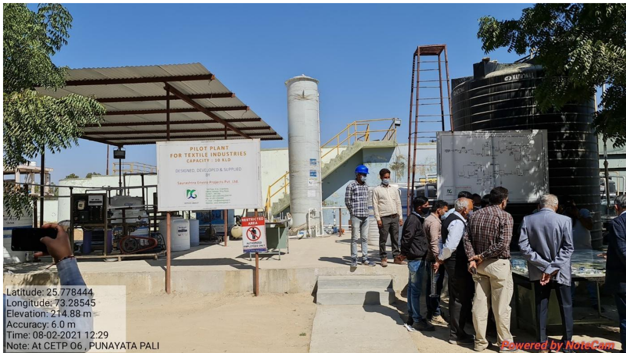
Fig. 2(w): Pilot plant of 10KLD for textile industries at CETP 06, Pali
