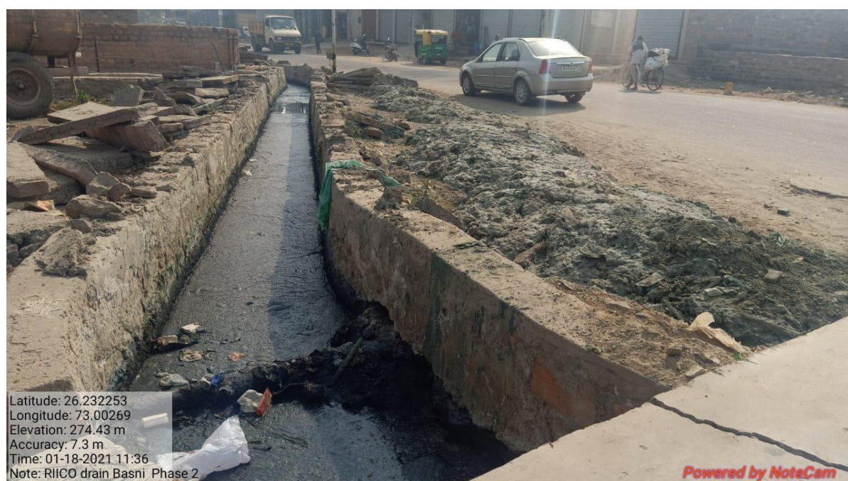
Fig. 1(f): Poor maintenance of Drain, Jodhpur
