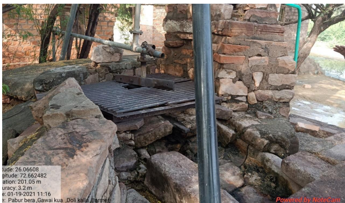
Fig. 1(o): Status of a well (Pabur Bera, Gawai Kua) which is now not being used due to contamination of water at Doli Village.
