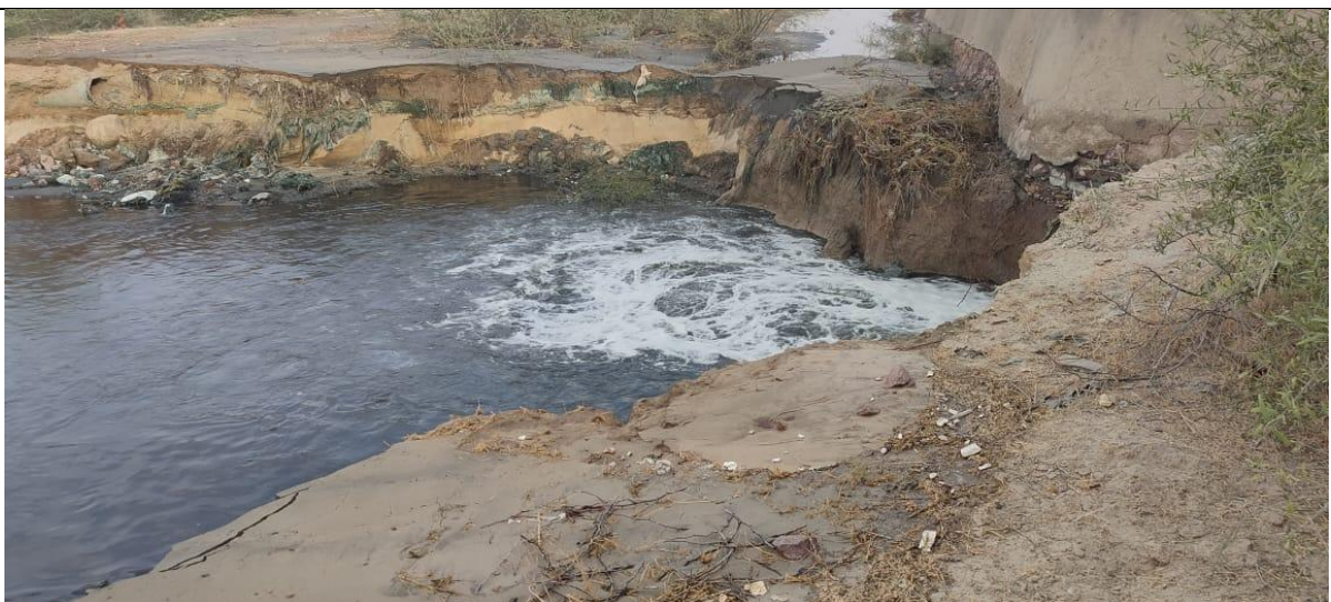
Fig. 3(l): Breach of SEP/HRTS, CETP Balotra on 22 March 2021
