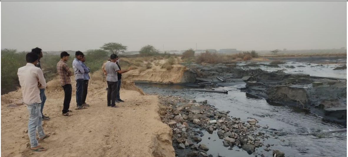
Fig. 3(j): Breach of SEP/HRTS, CETP Balotra on 22 March 2021
