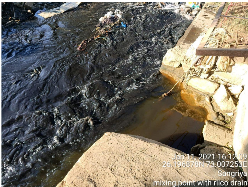
Fig. 1(k): Mixing point CETP Pipeline with drain, Jodhpur
